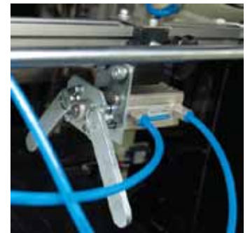
PLC Control Pneumatic Control Jogger
